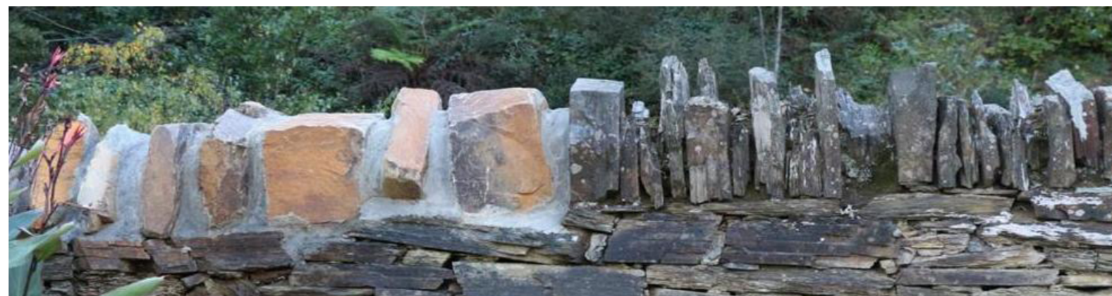
Figure 37: Repairs with cement mortar are inappropriate.
