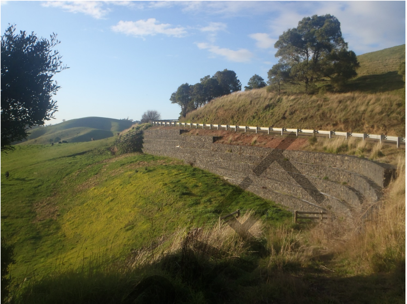
Figure 10: Examples of landslides repair on the road between Ferndale and Strzelecki.
